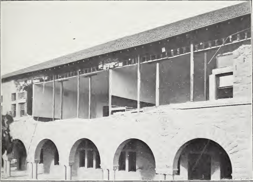
A. EARTHQUAKE DAMAGE DUE TO LACK OF TIE AND BRACING, GEOLOGICAL DEPARTMENT, LELAND STANFORD JUNIOR UNIVERSITY.
